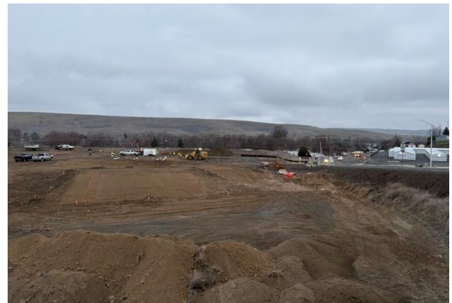
Construction crews working to install utility infrastructure into the development window. The ODFW office footprint is staked out in the foreground.
