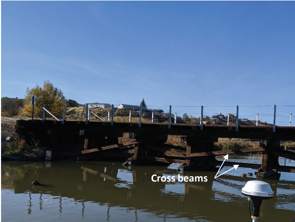
Figure 10. Site photo of the railroad bridge downstream of Lake Ewauna. Note that the piers are numbered to inform model input data. The cross, beams highlighted in the site photo, were assumed to be part of the bridge deck.
