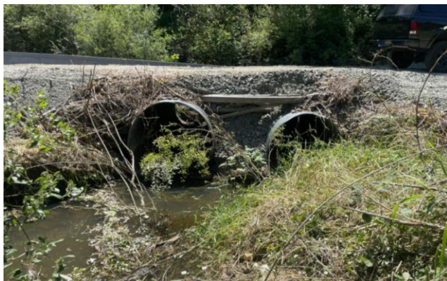
This culvert was impeding passage for adult steelhead and coho, particularly during low flows. Photo credit: Josh Hanson, ODF.
